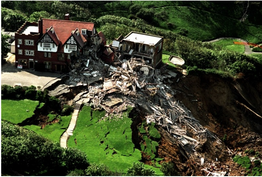
The scene at the Holbeck Hall Hotel in Scarborough after a massive landslide in October 1997.
